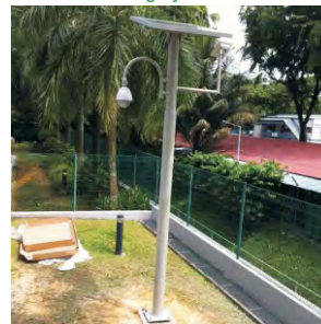
CCTV Monitoring System
