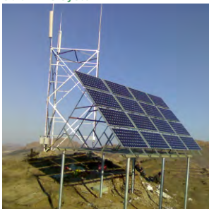
Solar BTS System
